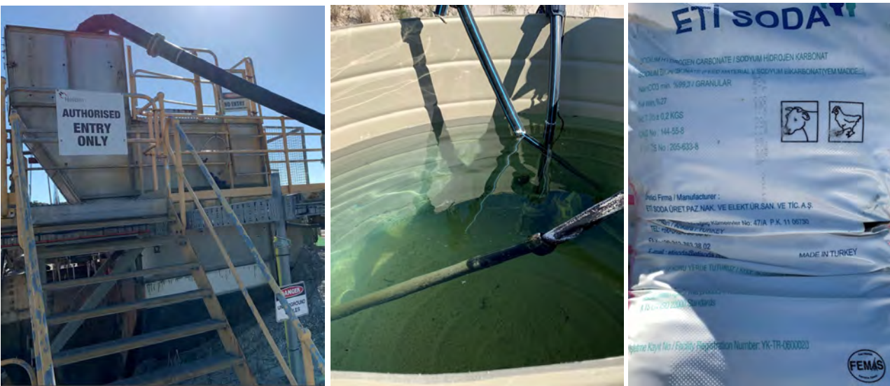
Figure 16 Wash screen, liming tank and bicarbonate
