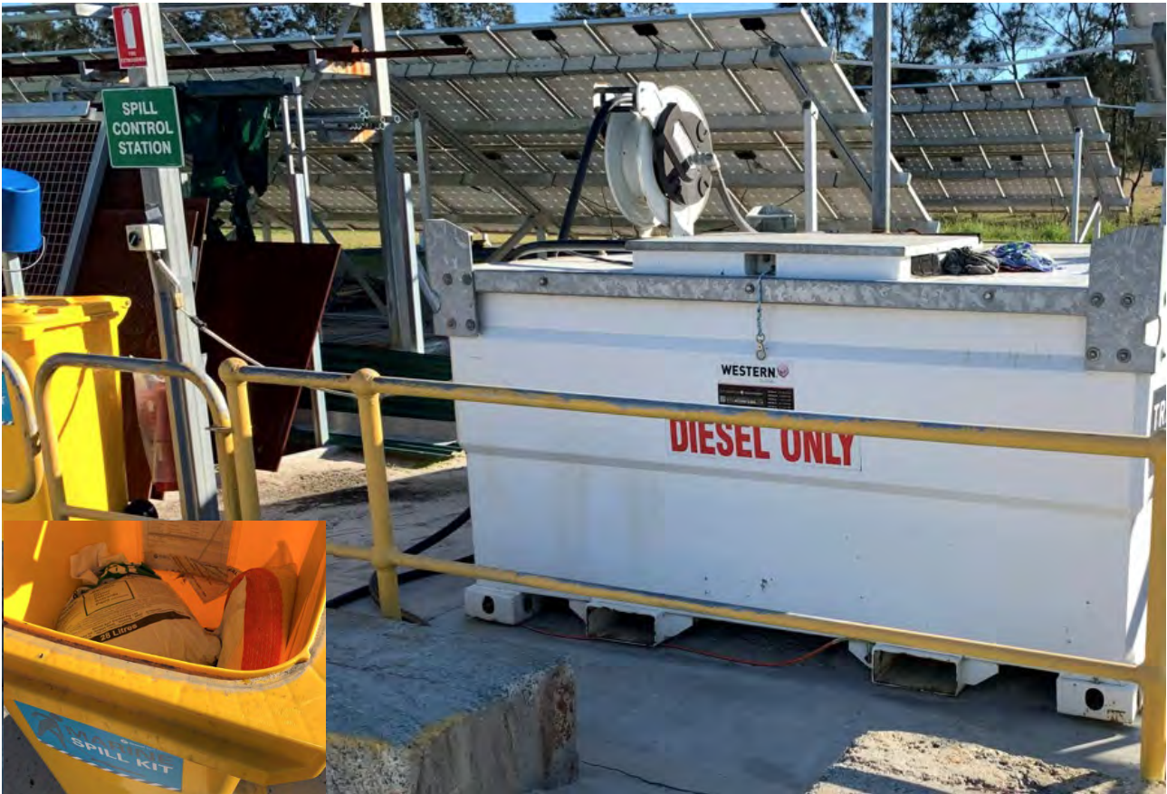
Figure 9 Bunded fuel storage and spill controls, solar power
